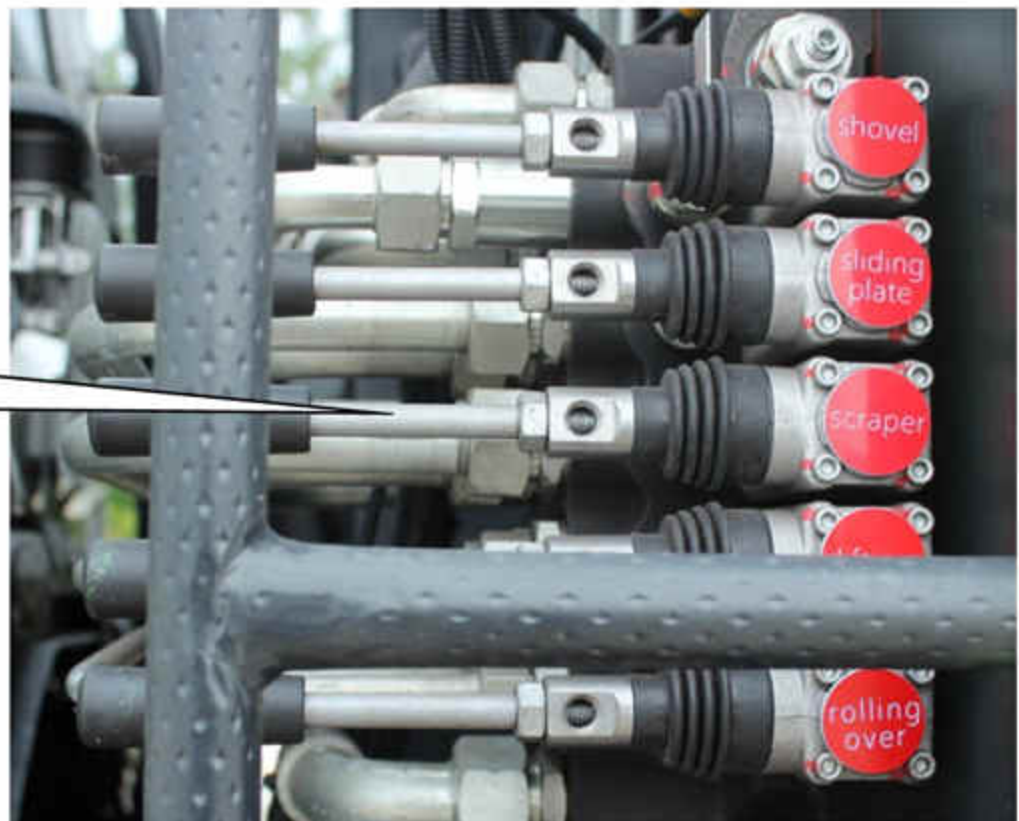
Hydraulic Control Joysticks (At drive side)
